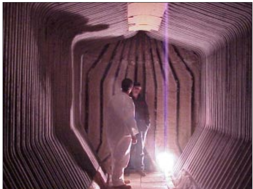
■ Inspection of boiler heat transfer surfaces after testing biofuels. The surfaces were almost as clean as after burning natural gas, and much cleaner than after burning No. 2 fuel oil.
