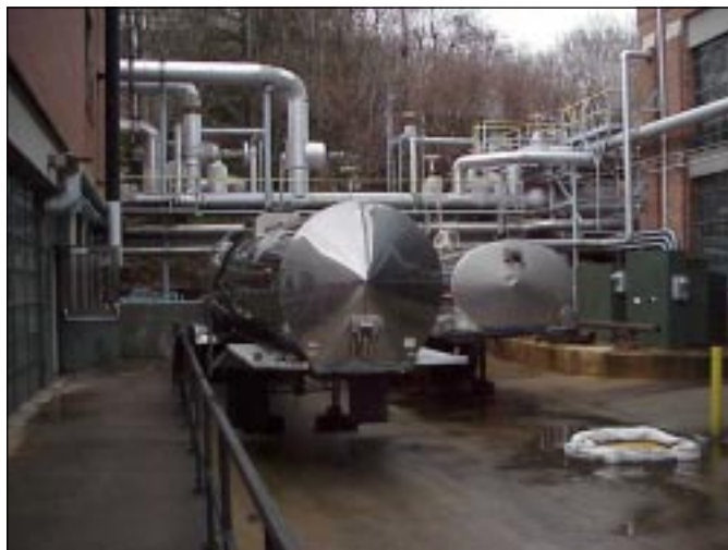
■ Tanker setup at the steam plant. One tanker was used to store the heated, recirculating biofuel while the other was used to transport the biofuel from the rendering plant to the university steam plant.
