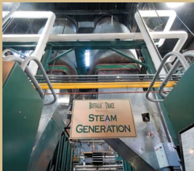
Above: Buffalo Trace steam generator. Opposite page: 1972 Erie City boiler.
